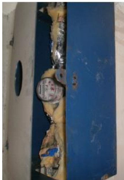
Picture 4. Water meter: Photo by Naira Harutyunyan
