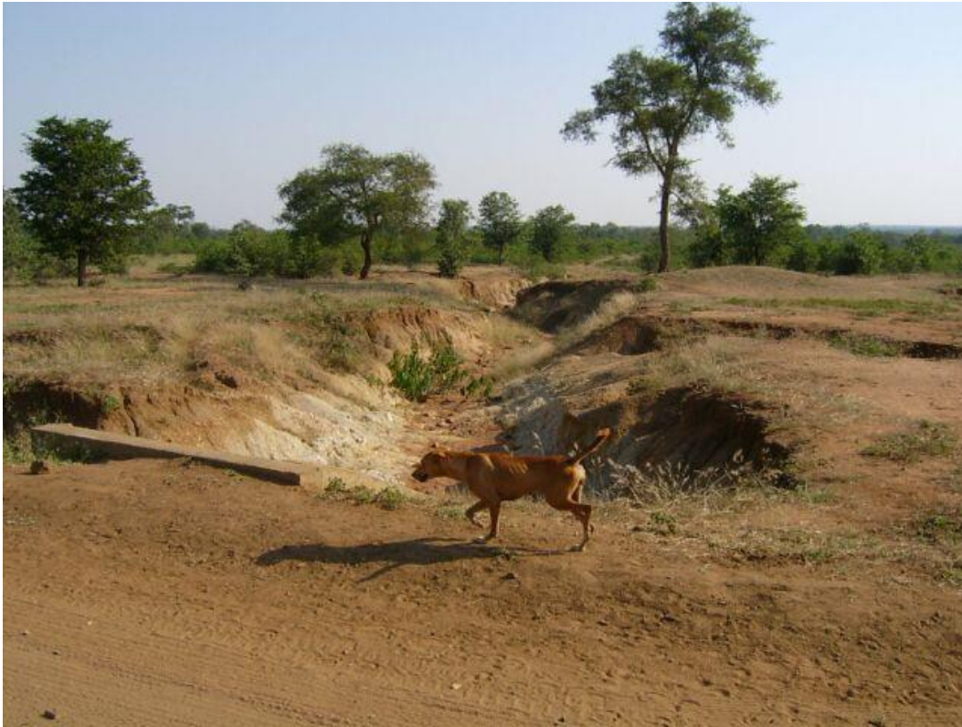
Figure 4.6: Drainage area near Jilongo village indicating soil erosion
