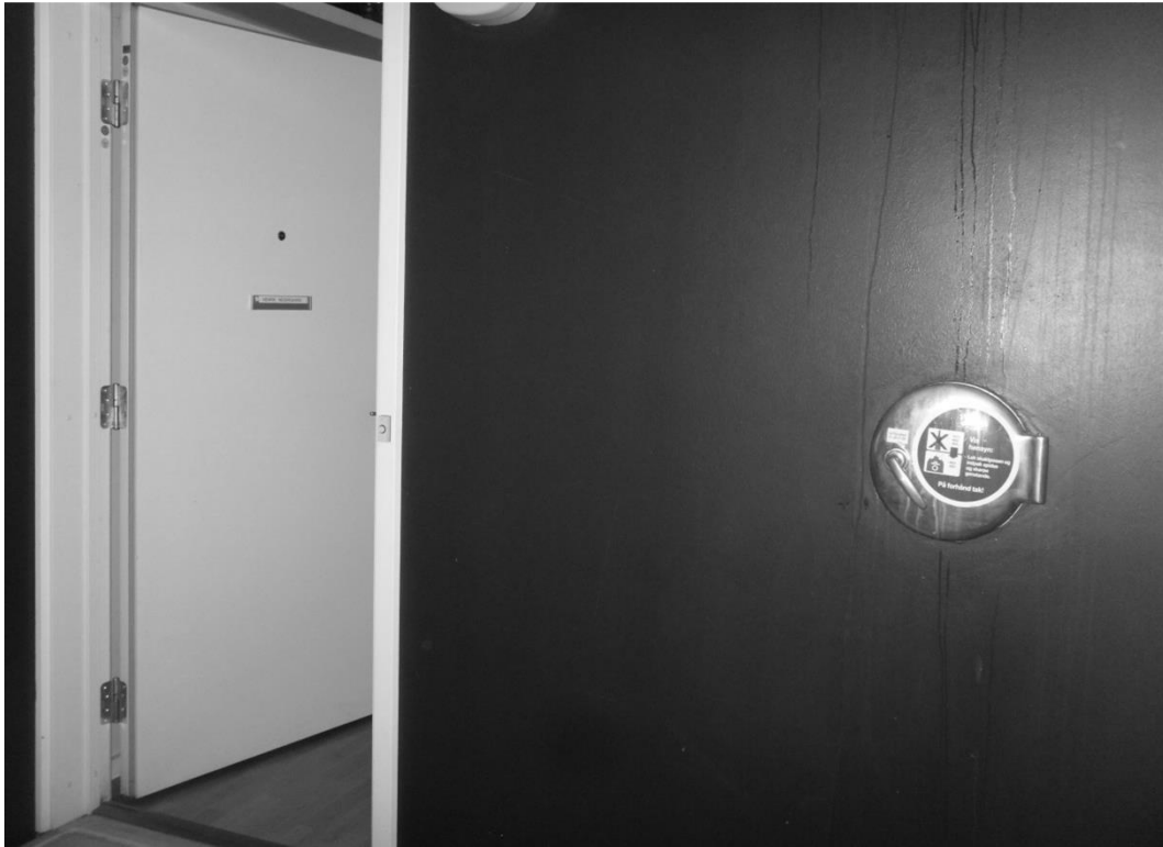
Figure 23. Waste Chute in an Apartment Hallway
