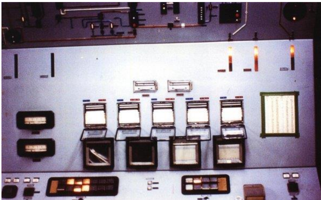
Figure 5.2 Control panel for lithium-6 production at Machon 2
