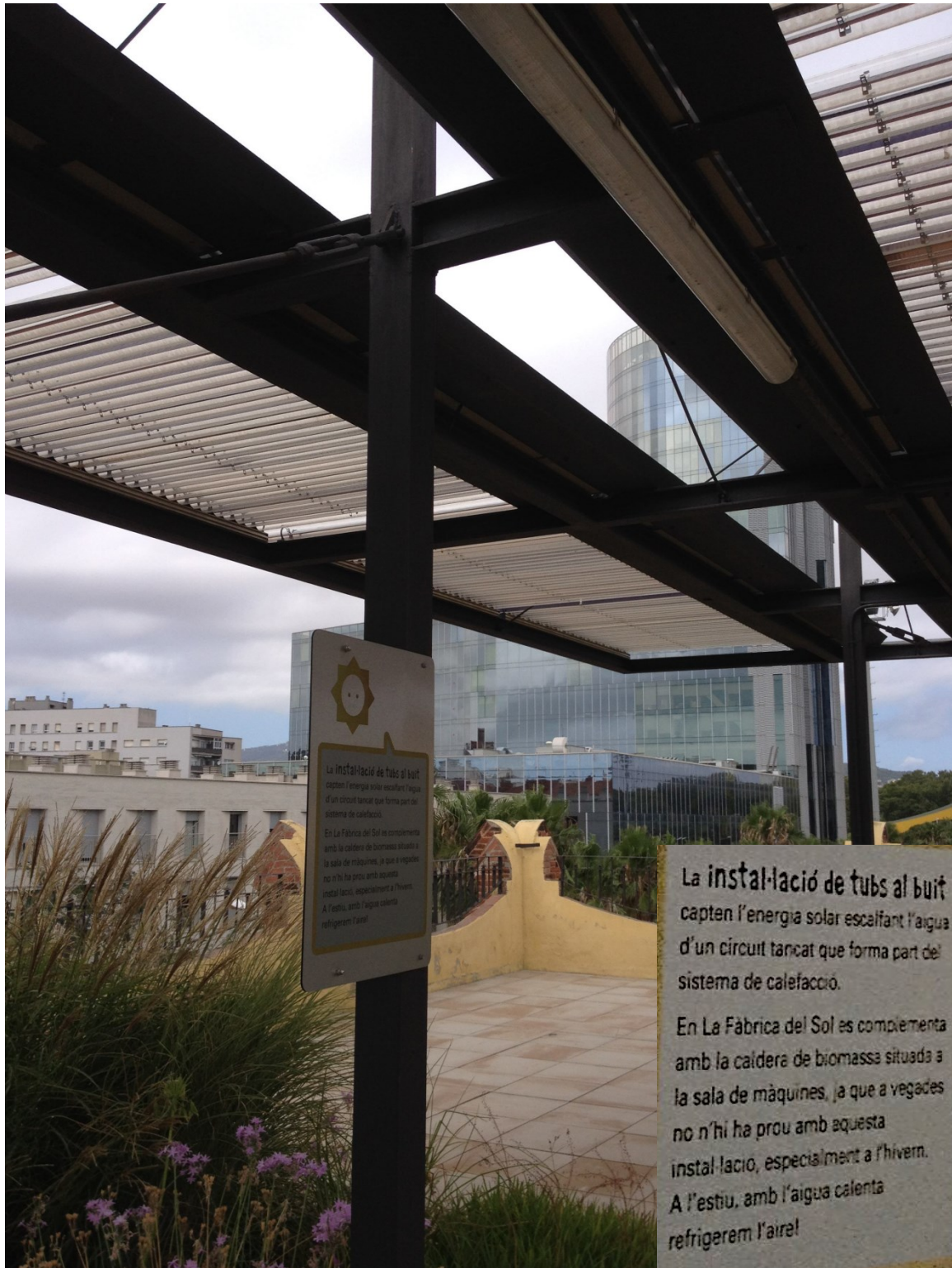
Figure 26. Solar thermal infrastructure on the rooftop of Fabrica del Sol , and information board indicating how this contributes to heating and cooling the building.
